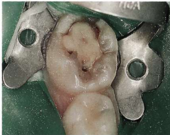
Figure 4.2 A failed glass ionomer restoration performed without complete removal of caries. The leaching of fluoride into the cavity does not stop the progression of caries.
